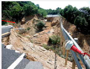
Collapse of a road embankment in the 2018 Japan floods (from Tsuchida and Hashimoto)
